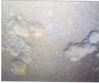
Corrosion damage on 10" pipe
