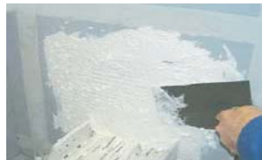
5.) Larger gaps and holes to be filled with mineral wool and covered with "A107".
