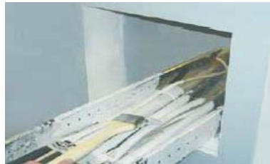
2.) ...and on cables (for a length of 300mm within the opening and 300mm outside it).
