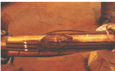
Filler & core damage
