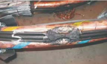
Filler damage, core intact
